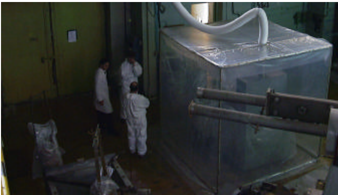
Fig.3.8 Tent with ventilation device for dismantling of radioactive wastes in reactor hall
